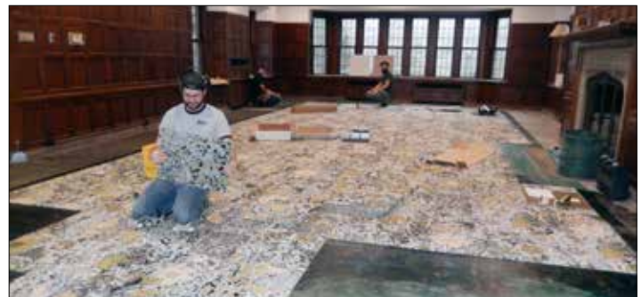
The laying of carpeting followed stripping and staining of woodwork, painting of walls and the installation of new ceiling tiles with recessed lighting.
